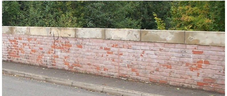
Unsuccessful anti-graffiti coating on a bridge in Leicestershire.
